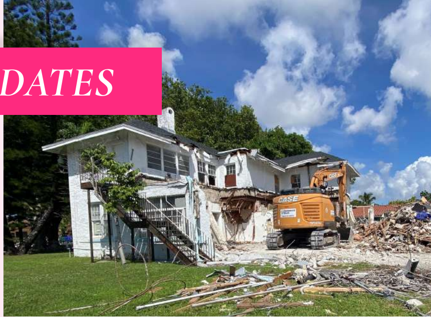
Residence at 1147 SW 13 Avenue that was given an unsafe structure violation and demolition order by the City of Miami. DHT is working with the owner to try to preserve this wonderful multi-family residence.
